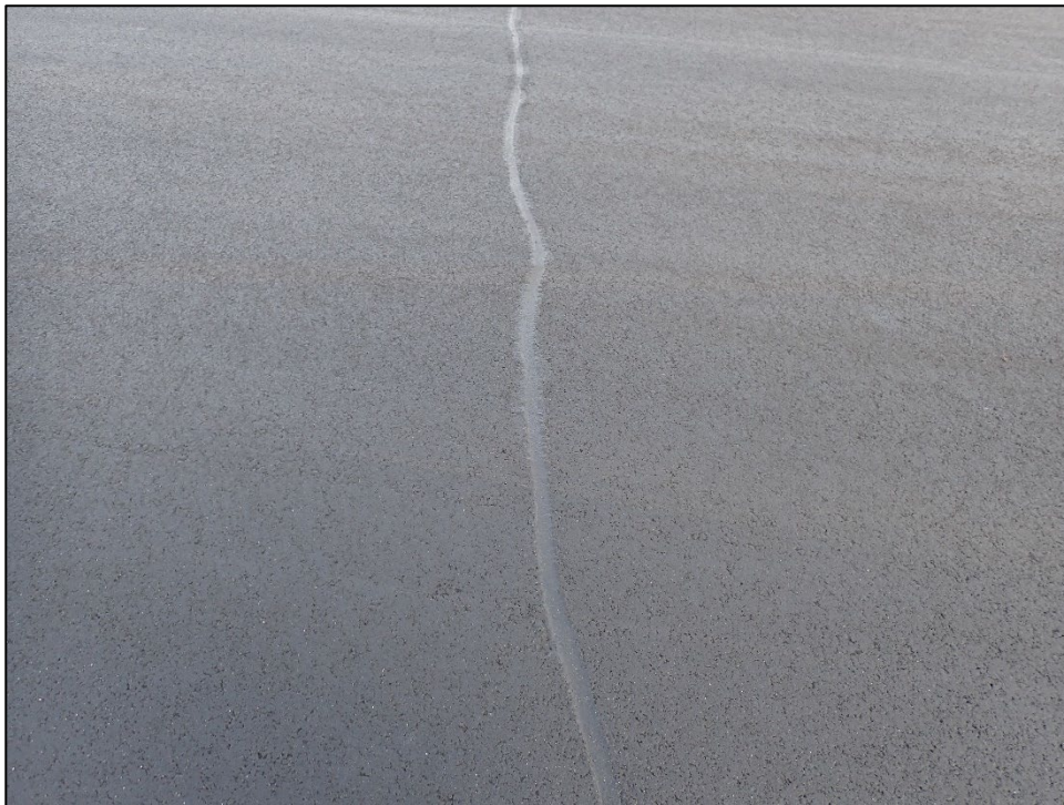
RW07-01-39: L&T Cracking
