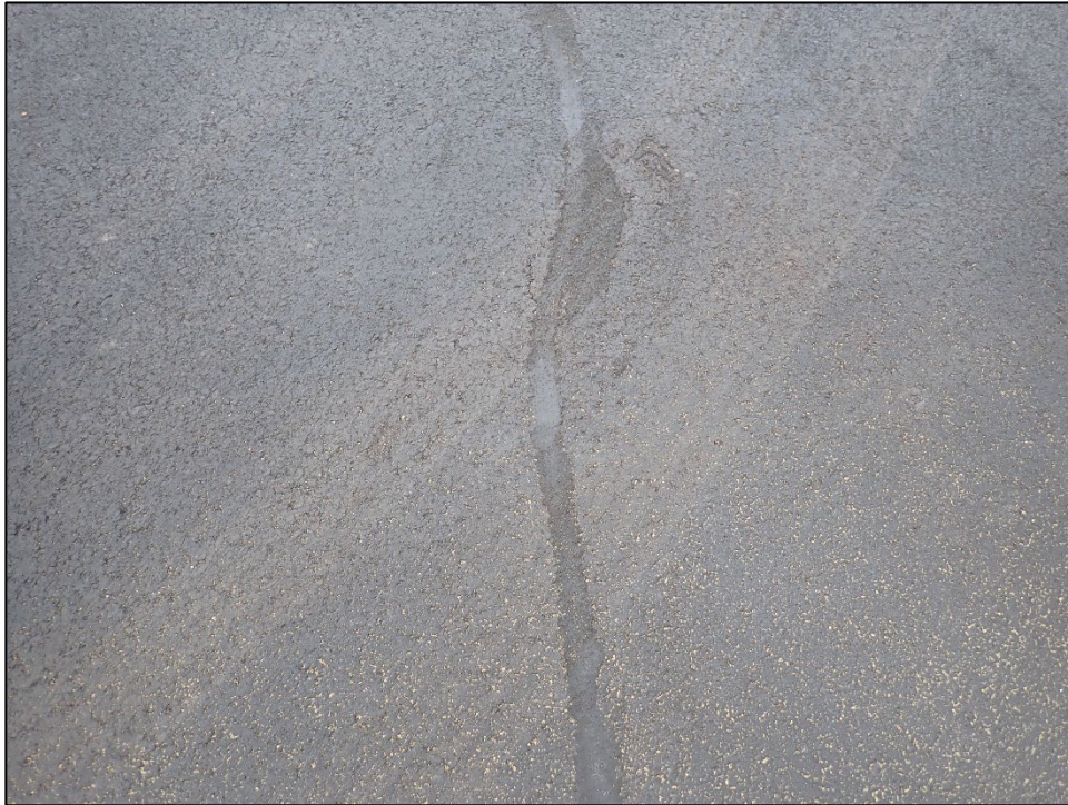
TW-01-02: L&T Cracking
