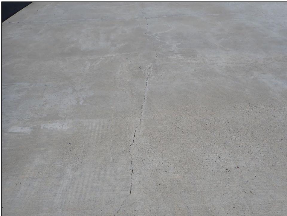
AP-02-01: LTD Cracking
